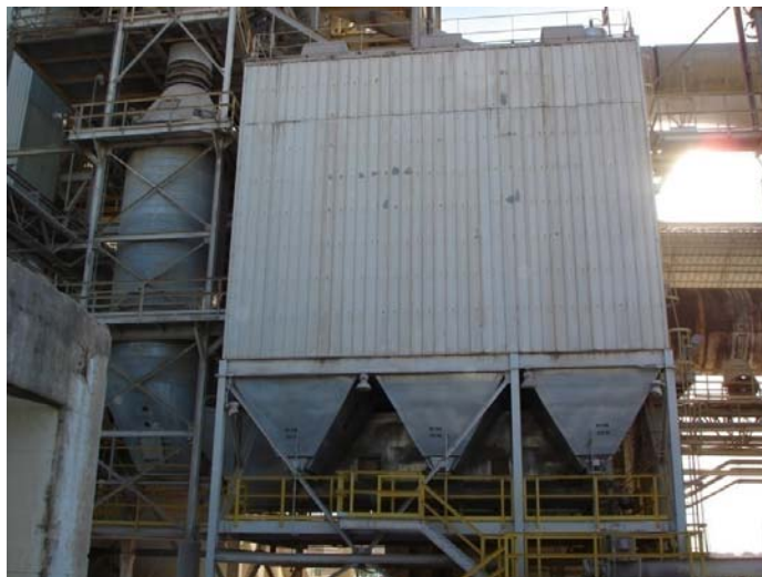
Figure 1- Dust control device (Courtesy of Capitol Cement)
