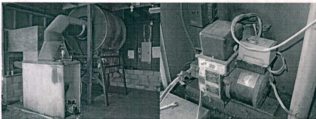
Figure 2.3 Diesel Dryer, 1,600 dried lb and its propane burner and Interchanger
