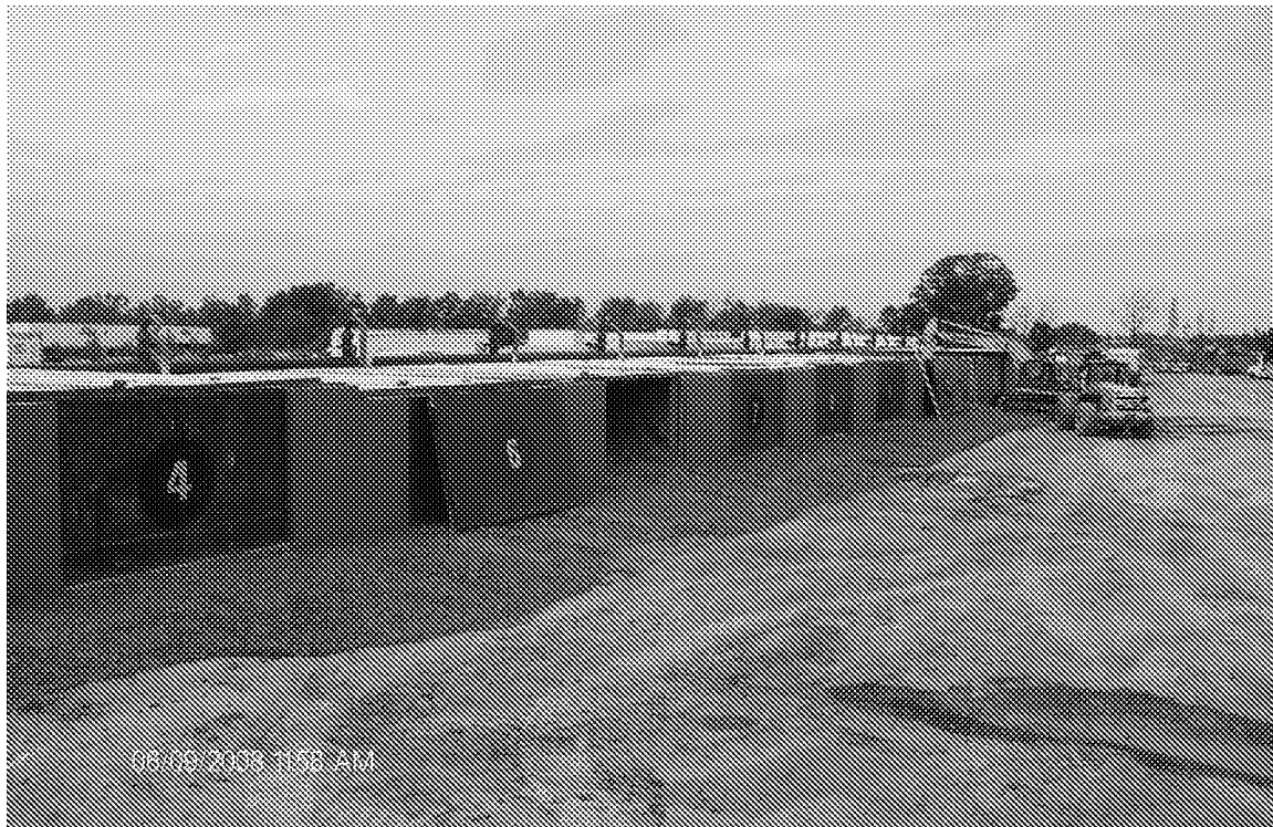
View of treatment cells 4 to 14.
