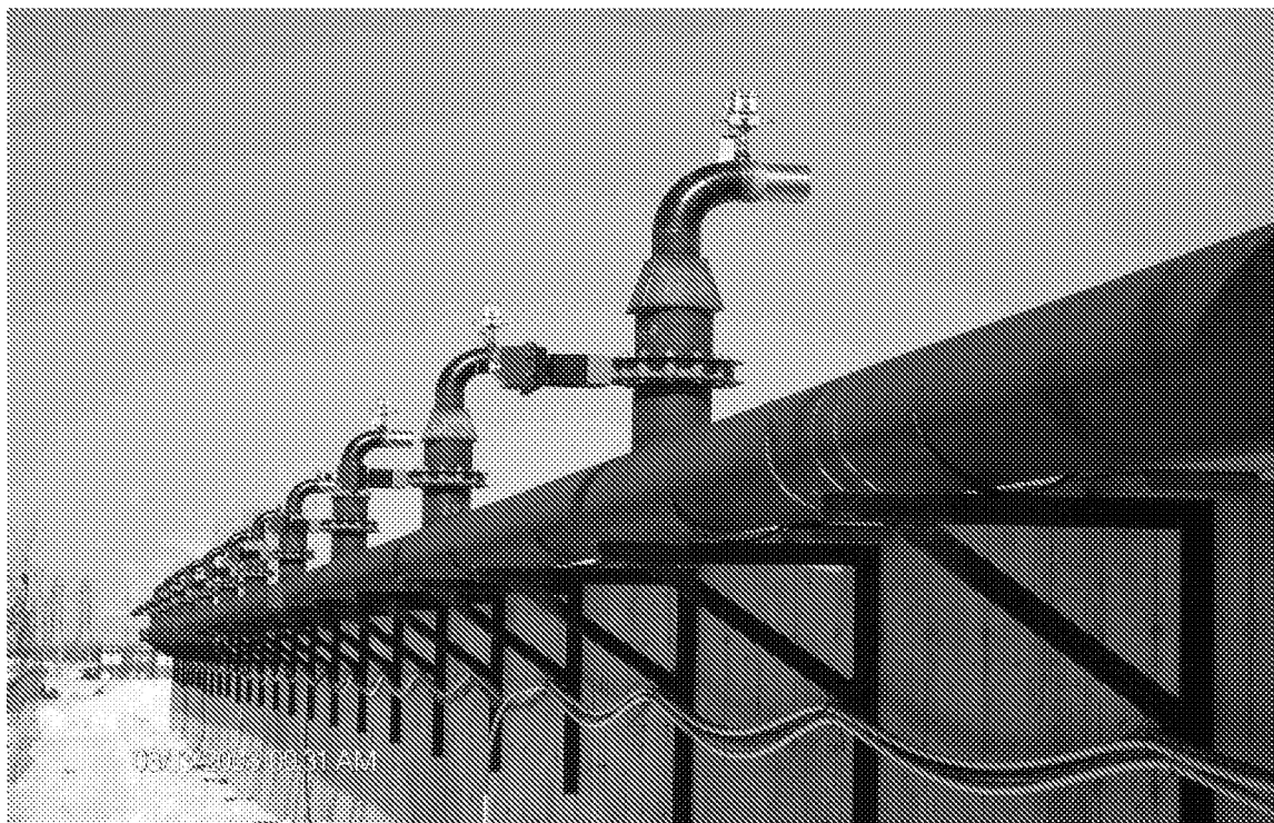
Vacuum extraction infrastructure above the treatment cells.
