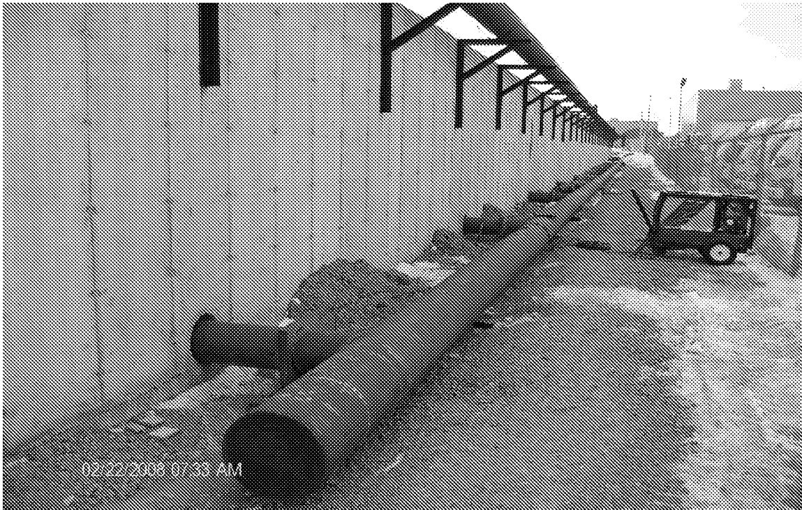
Heat distribution system at the bottom and vacuum support infrastructure at the top.
