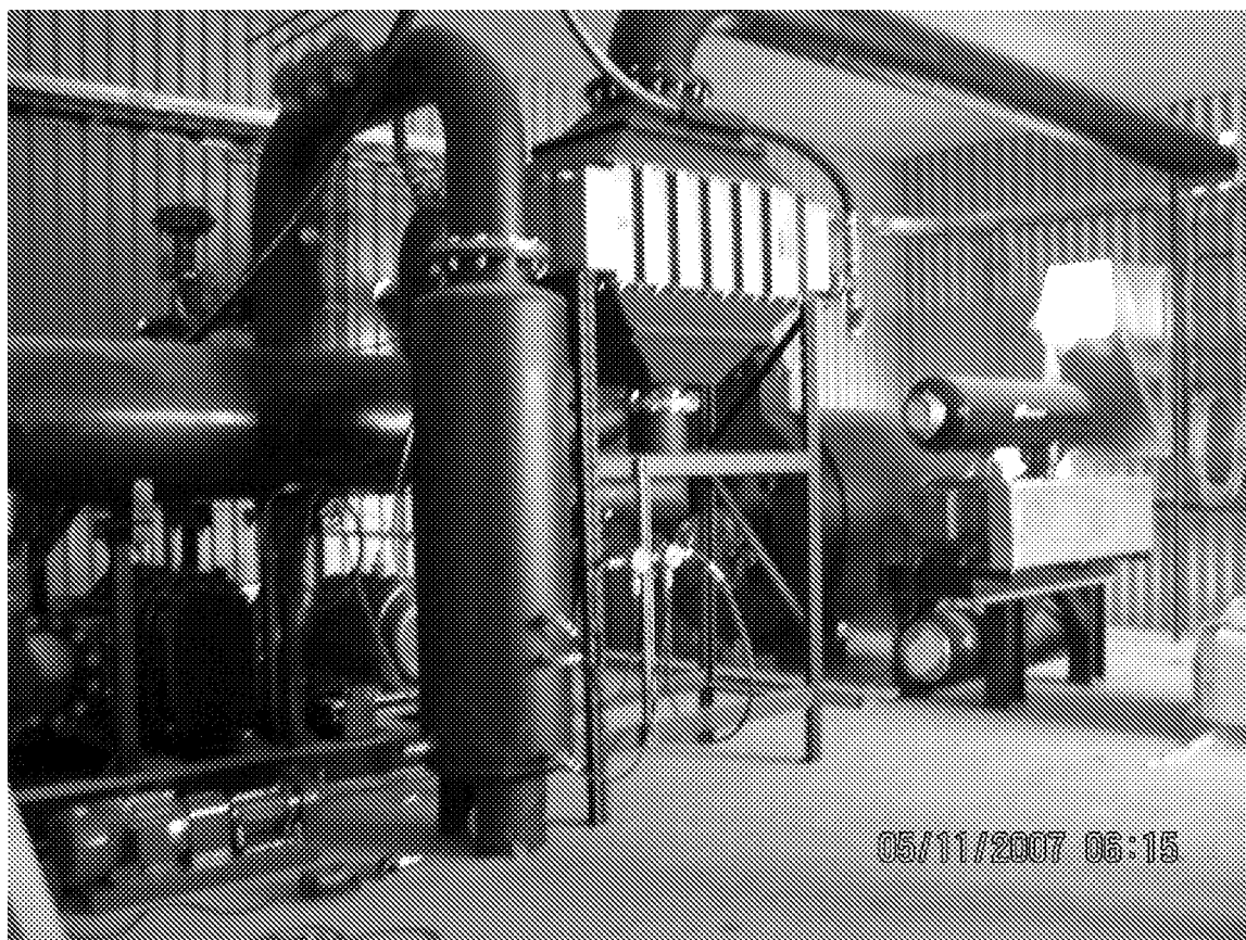
The mechanical room: a vacuum pump on the left, a condenser in the upper middle section and a liquid condenser tank in the middle, a heating furnace on the right.
