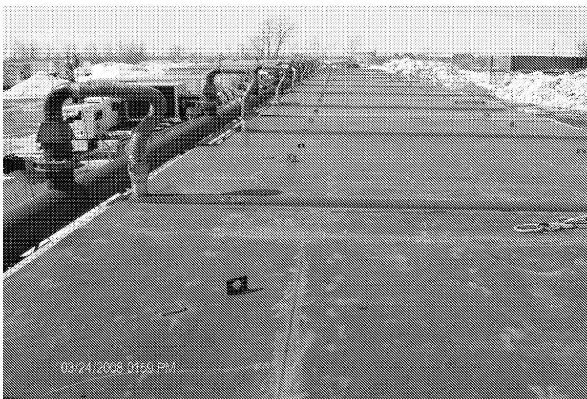
The steel roofs and vacuum application manifolds above the cells with isolation valves on each conduct.
