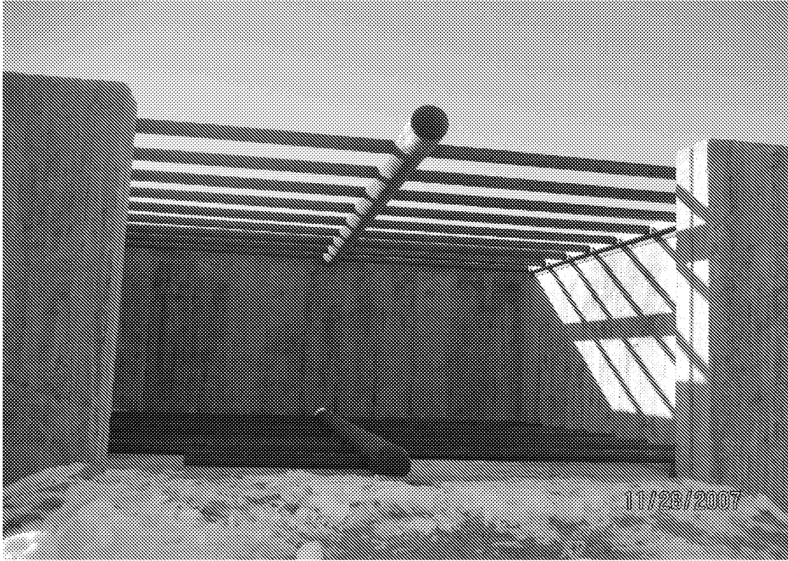
The hot air distribution system at the bottom and the vacuum-related pipes at the top. The top infrastructure is incorporated to the roof structure when built.
