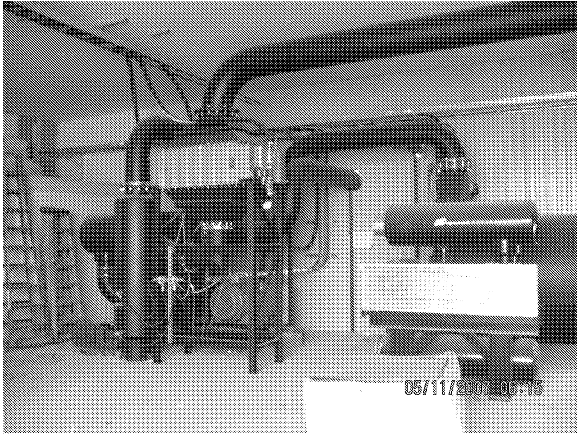
Side view of the mechanical room.
