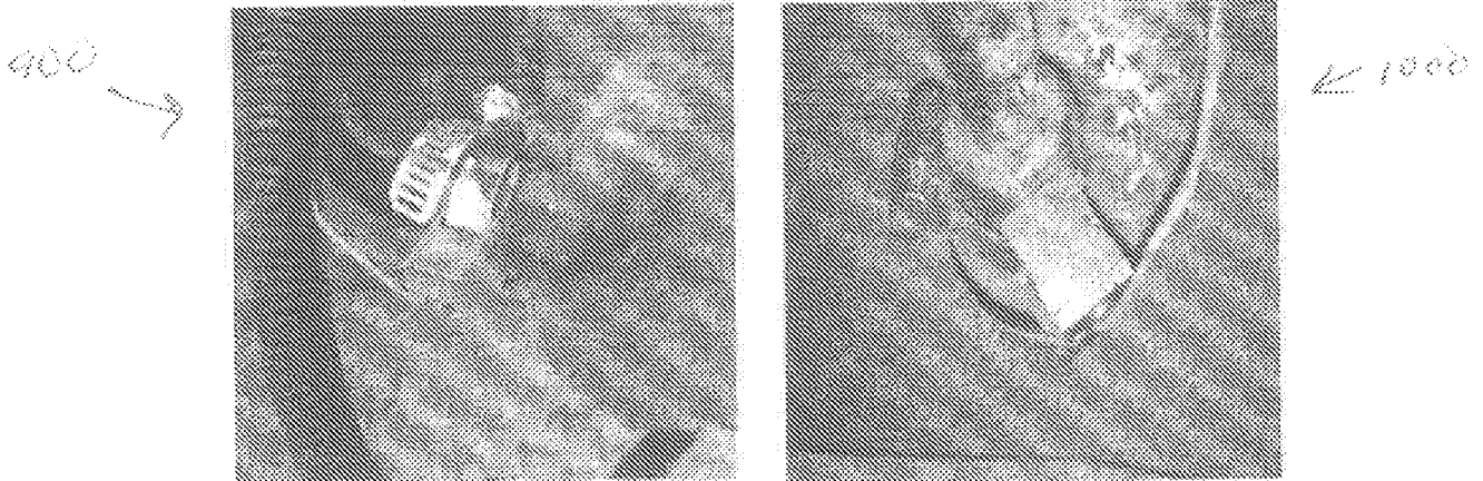
Sensor installed on fuel suction and return line
