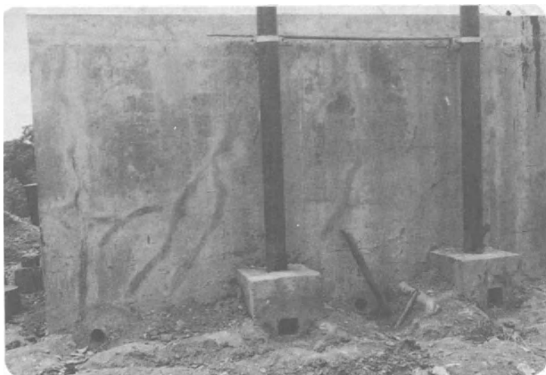
Photo 4 Side view of kiln with two smoke pipes and air inlet holes at the bottom. Ghana. (Photo W. Emrich)
