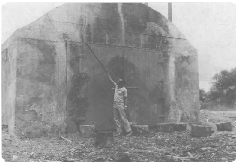
Photo 3 A Missouri kiln. The shell is dangerously cracked as a result of faulty operation. Ghana. (Photo W. Emrich)
