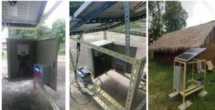
Figure 5. All electronic devices are put in a waterproof control box.
